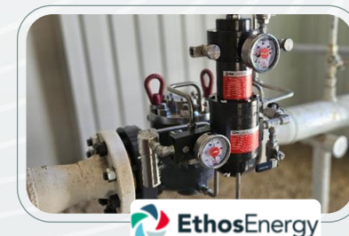
PG&E Trenton Station Ethos Energy
